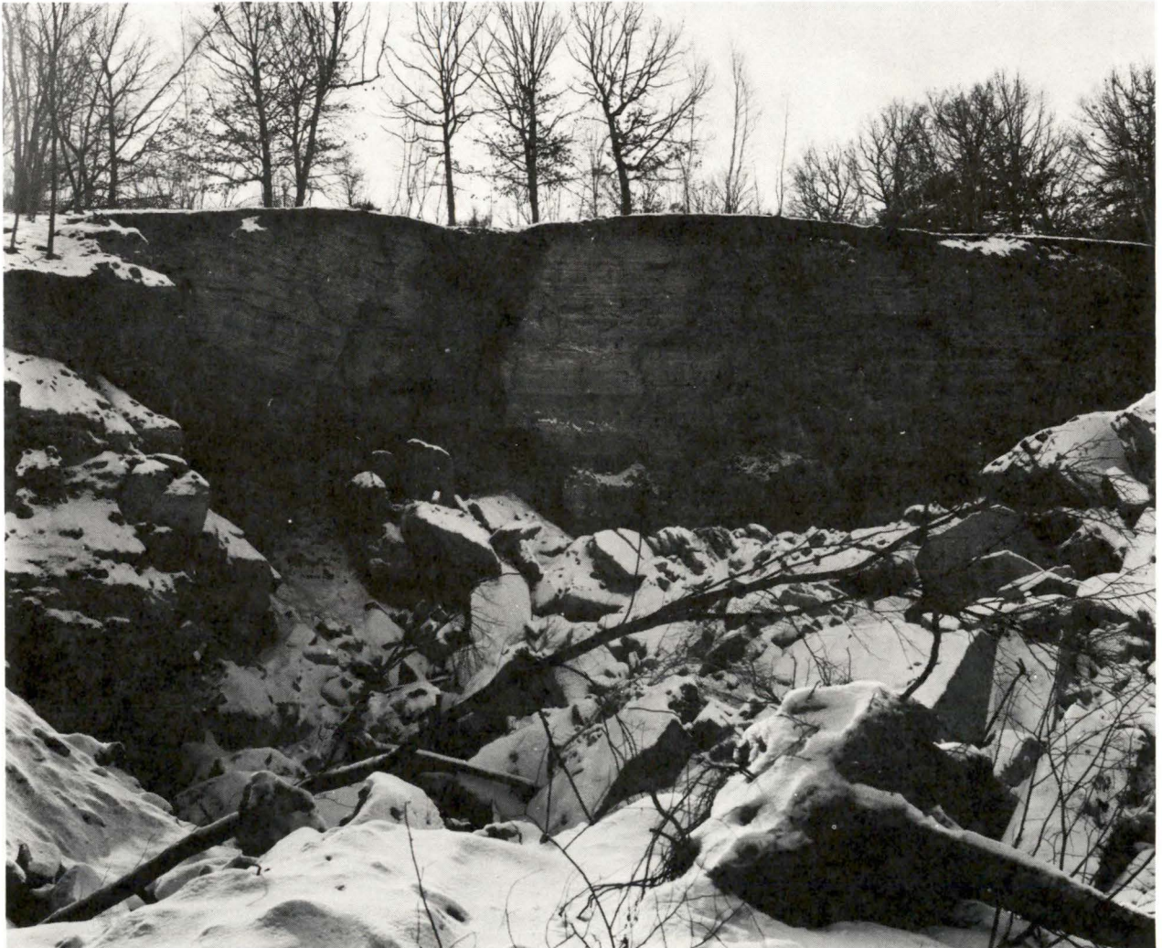
FIGURE 18. - View of soil cover over south end of failure.
