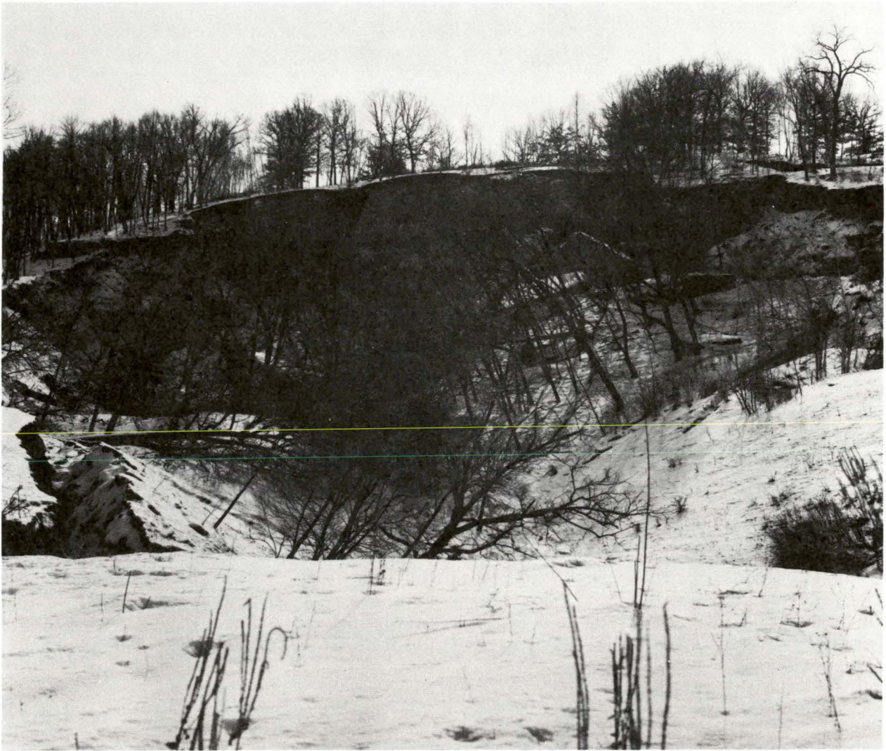
FIGURE 1. - Surface failure over the Batsch mine looking south.
