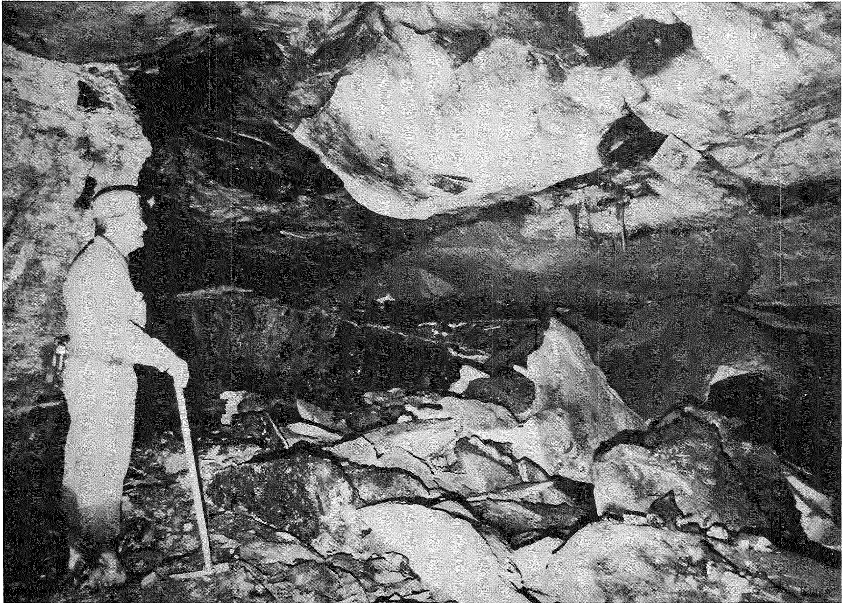
FIGURE 21. - Hazardous roof conditions in 6-West section at heavily slickensided washout contact. Fallen rock consists chiefly of argillaceous sandstone.
