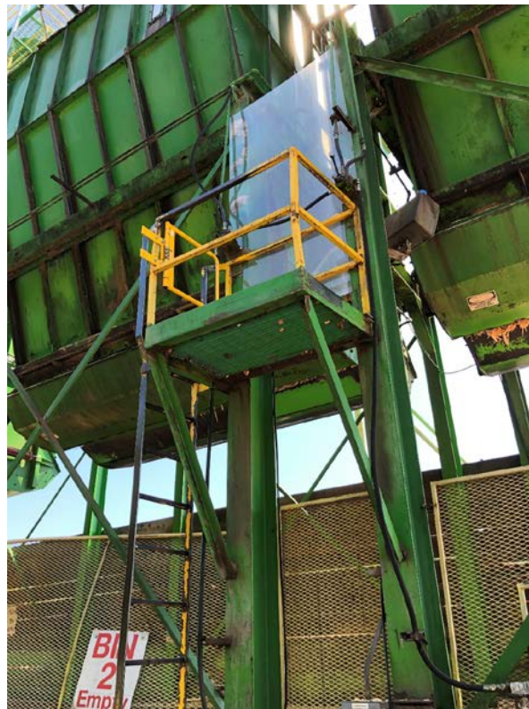
Photo 9: Bin control platform with ladder that truck drivers used to access hydraulic levers for clamshell gates that released woodchips into the trailer.
