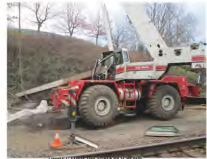
Figure 1: Crane cab struck by H-beam.
