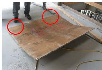
Plywood cover that failed. Circles indicate the two nails that secured the cover to the stem wall sill.
