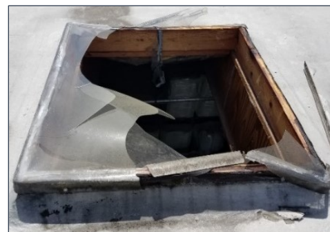
Skylight the roofer fell through.
