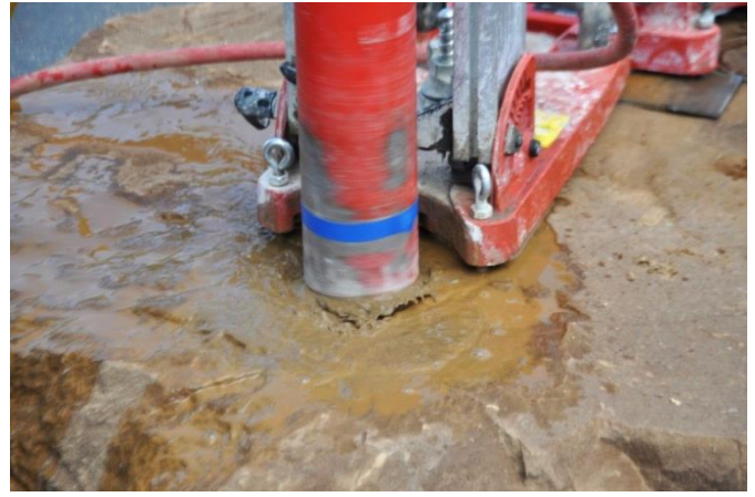
Fig. 15. The core bit is drilled to the depth of the blue tape.
