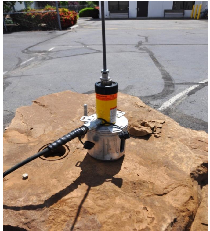
Fig. 19. The hydraulic ram pushes upward against a nut attached to the all-thread that is in turn connected to a pulling bolt anchored in the test core.
