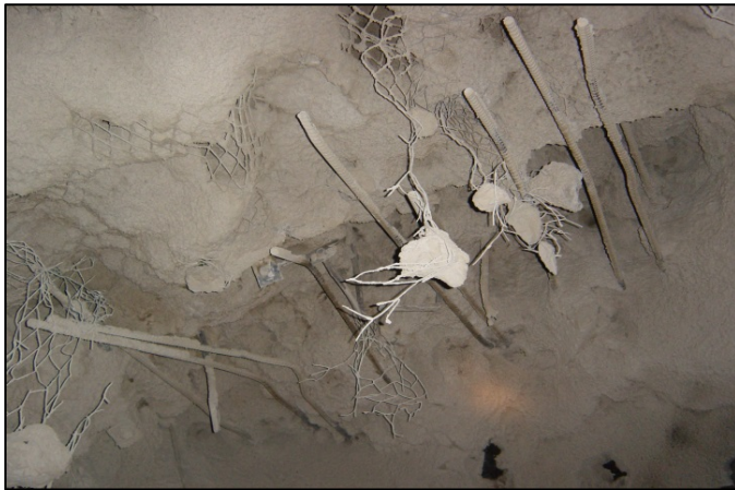
Figure 3. Ground failure in a high yielding underground mine.
