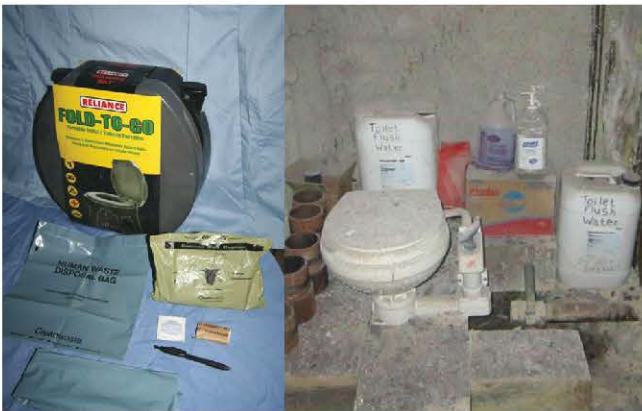
Figure 4: Examples of toilets in a bag that can be used on their own or with a collapsible toilet (left). Separate toilet room constructed by the mine (right) with marine-type flushable toilet and associated flushing and sanitizing products.
