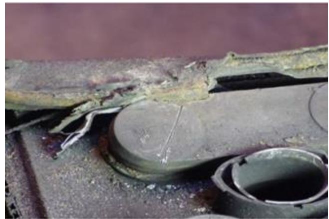
Fig. 1. Scoop-tractor battery showing terminal contact with steel battery tray.
