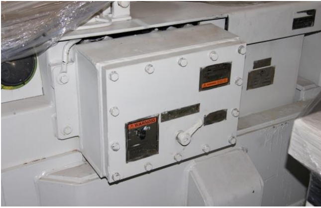
Fig. 8. Side-mounted battery circuit breaker box.
