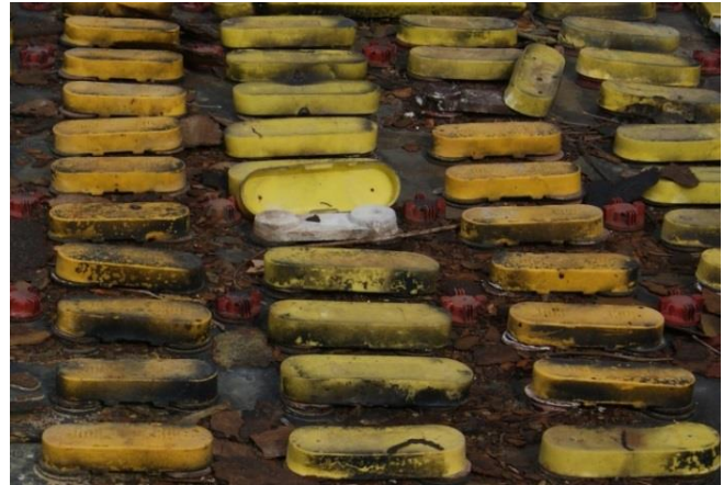
Fig. 9 Debris and leakage buildup on terminals.
