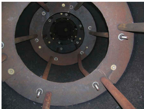
Figure 5 Initial baffle system that failed.
