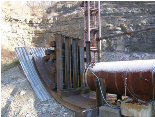
Figure 7 Silencer at the exit of GETF.
