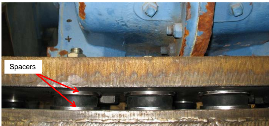
Fig. 12—Spacers installed above and below the top portion of the vibration isolators.
