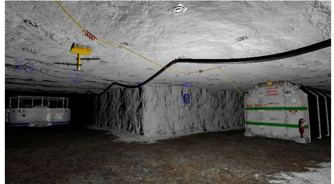
Figure 2. Examples of the mine phone, leaky feeder, and mesh node 3D art assets for communications systems implemented in VR Mine, where the blue boxes along the cable also represent communication network nodes and the green box represents the mesh network nodes.
