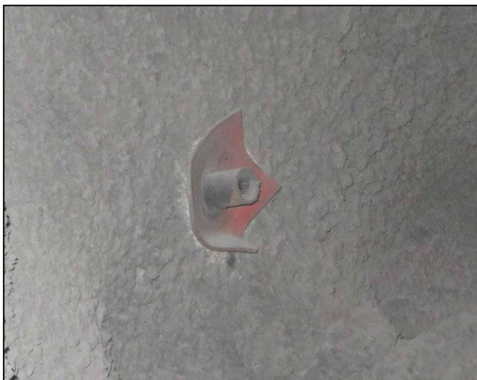
Figure 3. Bolt head beginning stages of popping off.
