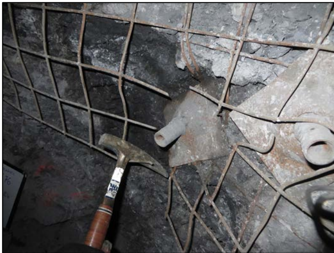
Figure 2. Bolt head pulled through welded wire mesh.
