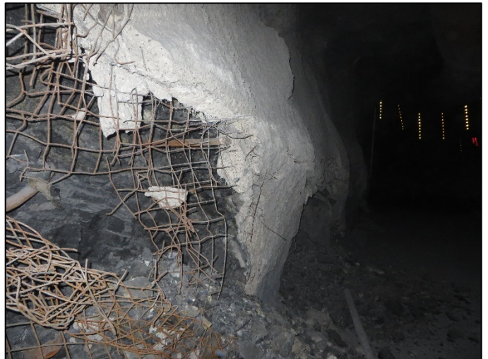
Figure 5. Buckled shotcrete rib.
