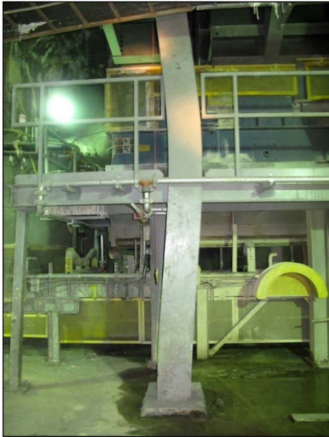
Figure 6. Bent structural beam in critical infrastructure caused by convergence (Internal mine memo).
