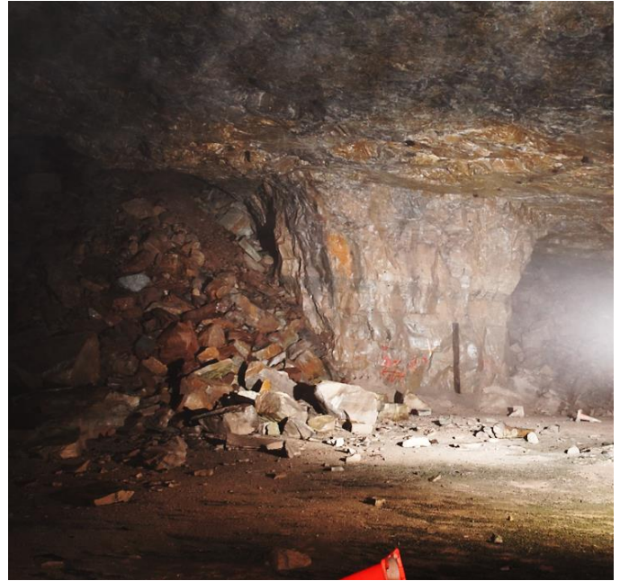
Figure 7. Rubble from the roof collapse and a stable pillar along the edge of the benched area that collapsed.
