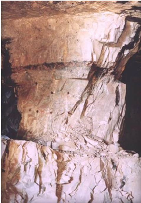
Figure 5. A pillar impacted by large angular joints along the edge of bench mining (photo, by A.T. Iannacchione).
