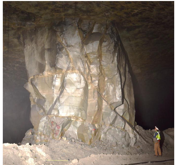
Figure 3. Prominent N60°W striking joint intersecting a pillar south of the collapsed area.
