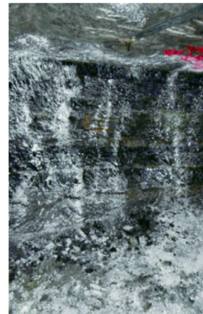
Fig. 12. Observed rib conditions at Site 2.
