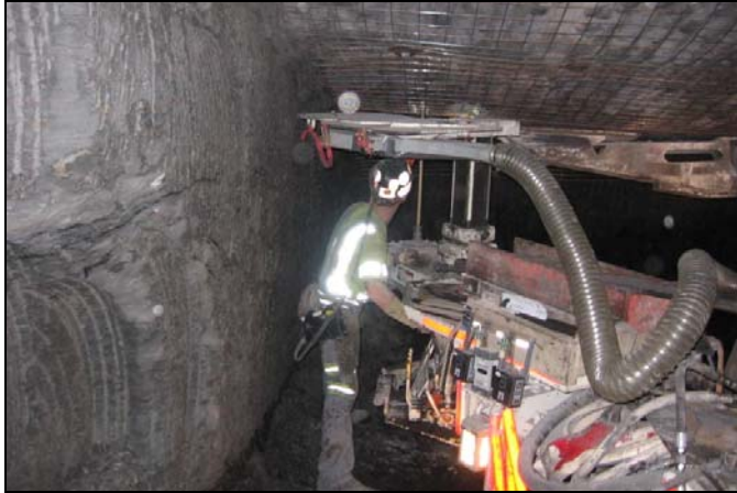
Figure 15. NIOSH-designed air canopy system on roof bolter in underground coal mine.
