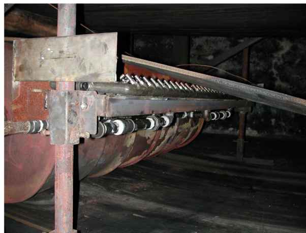
Figure 3 — Natural gas burners to ignite belt.
