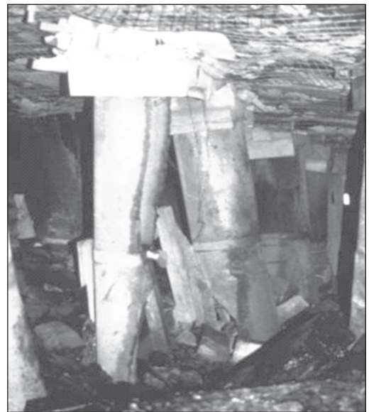
Figure 14. Failure of high capacity concrete crib in longwall tailgate
