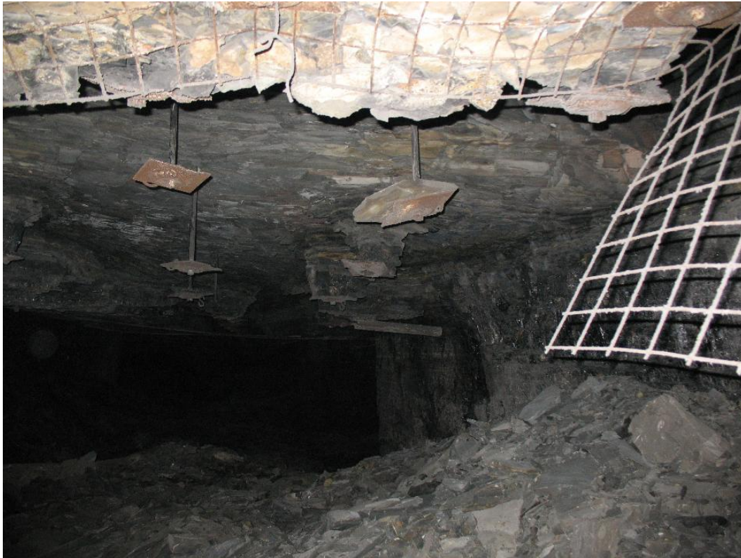
Figure 20: Progressive roof spalling leads to roof fall.
