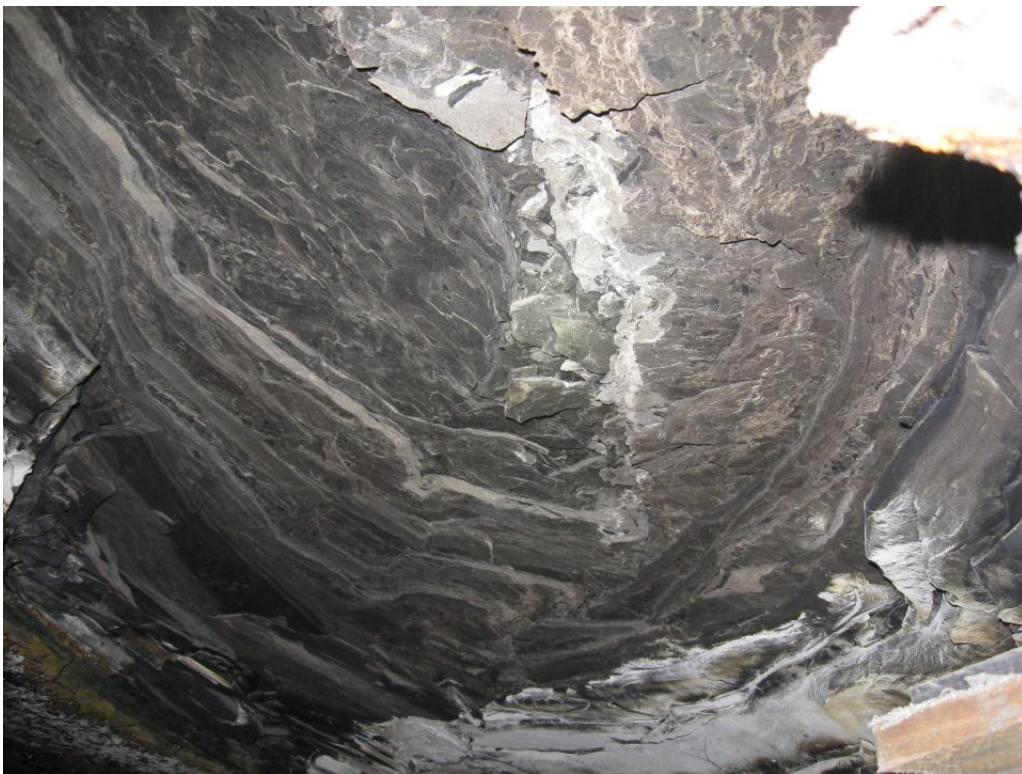
Figure 16: Roof pot and rock stitching caused by horizontal stress.
