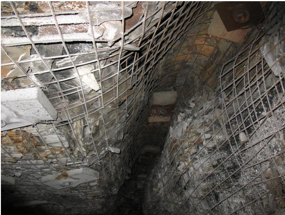
Figure 33: Screening of rib gutters can stop further deterioration.
