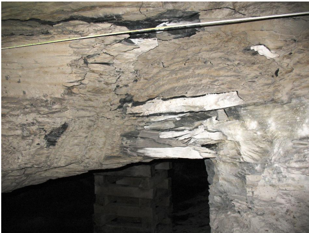
Figure 42: Stairstepping fractures extend over the pillar.
