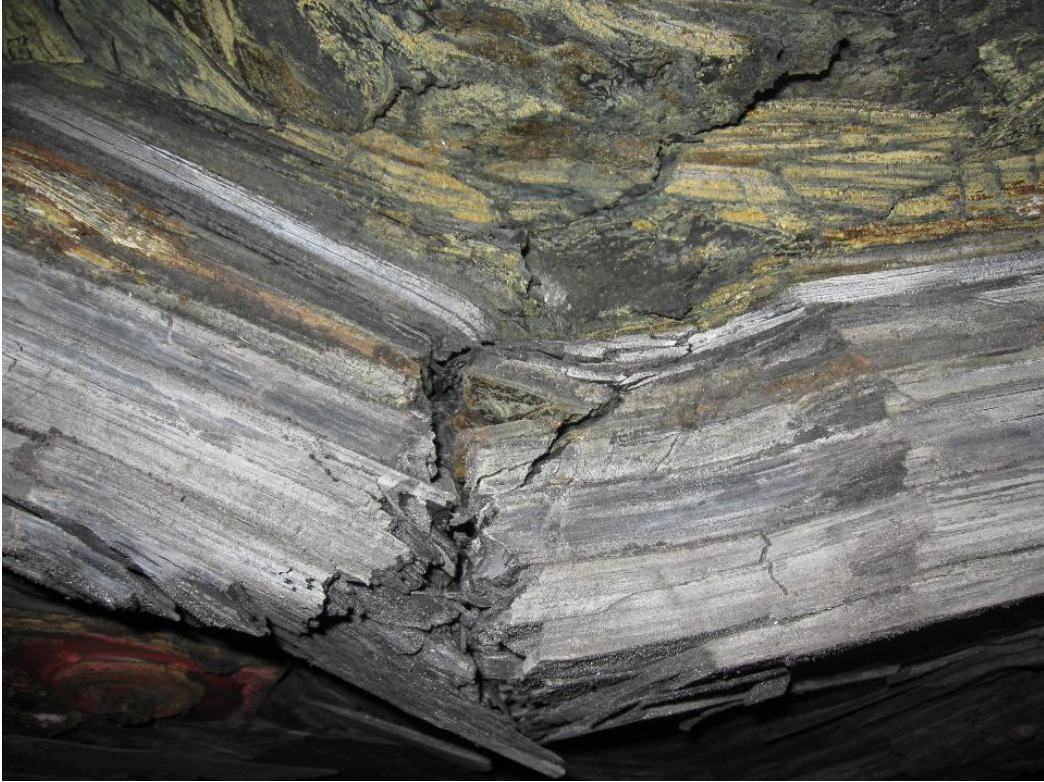
Figure 39: Tension crack develop in entry center as roof sags.
