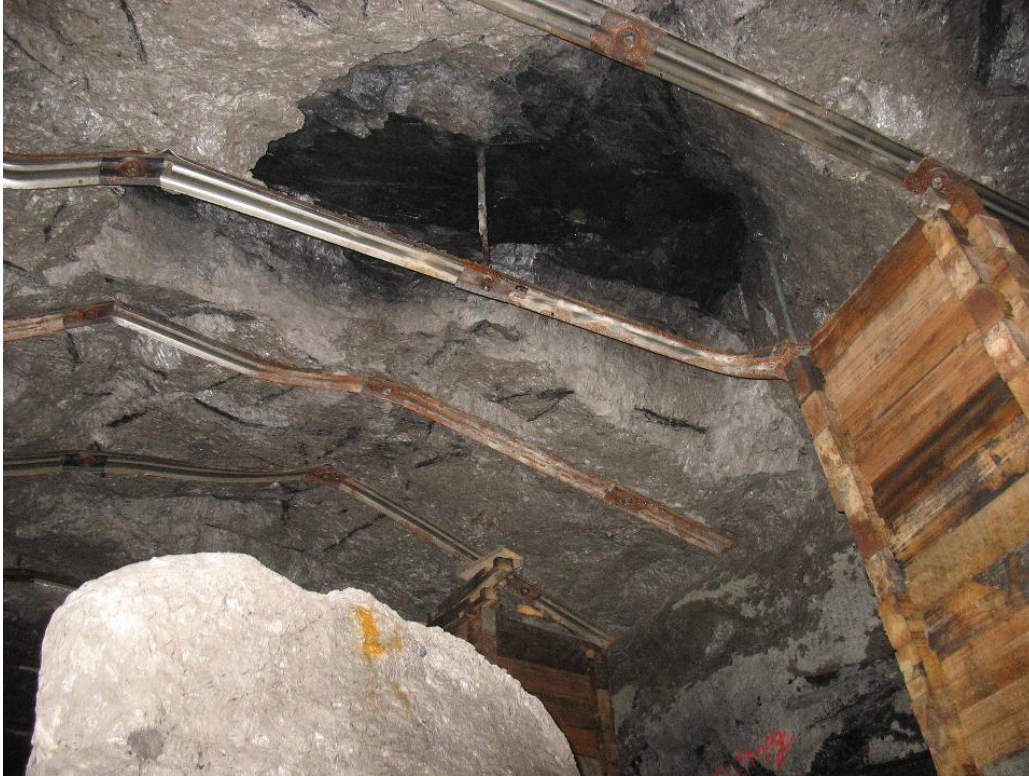
Figure 21: Weak cohesion in a roof fireclay leads to fall between bolts.
