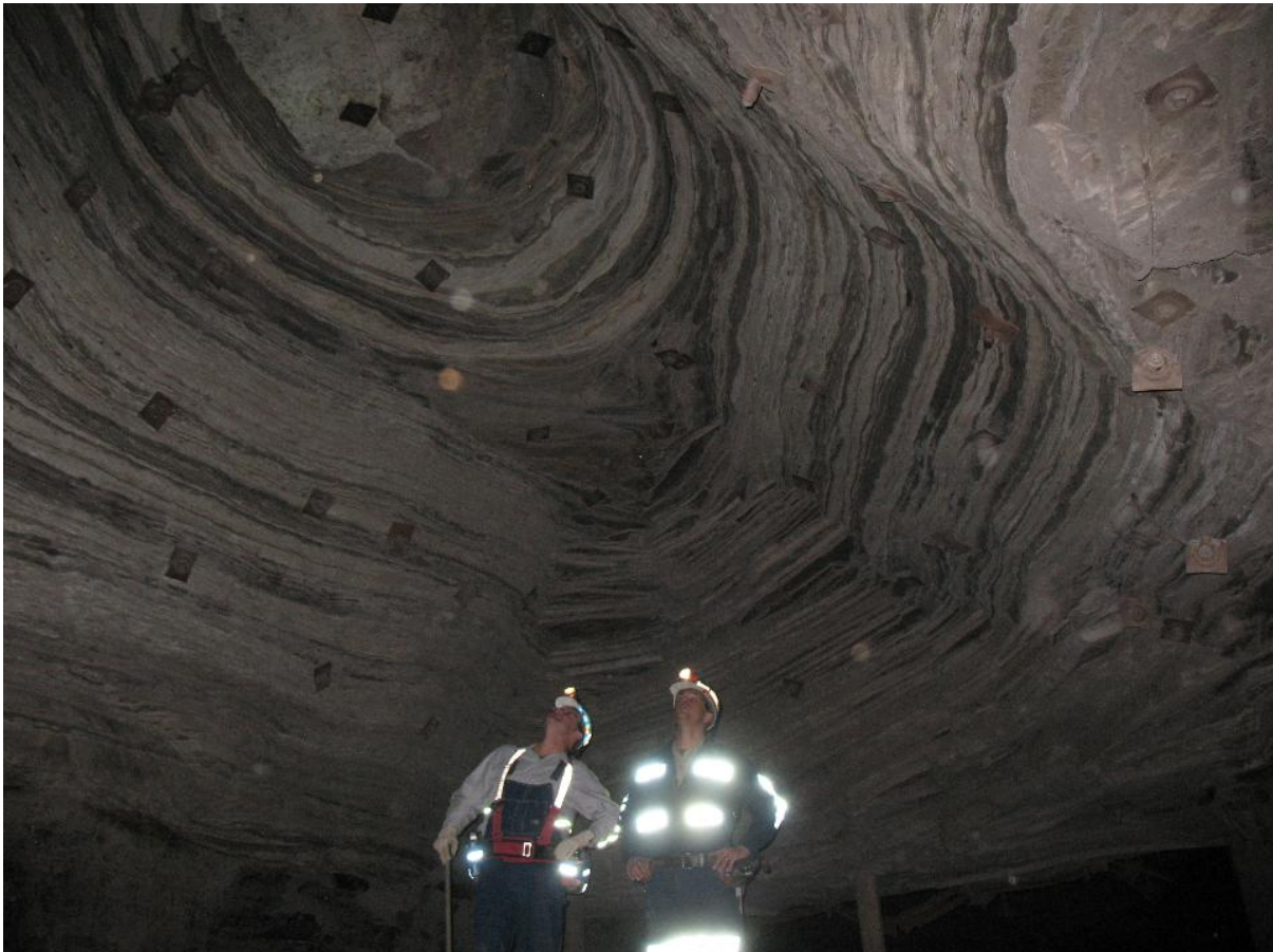
Figure 1: Roof fall in a stackrock sequence.
