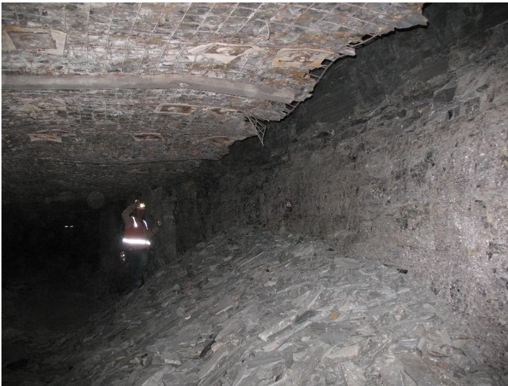
Figure 23: Rock pile below rib gutter is due to disaggregation of weak roof shale.
