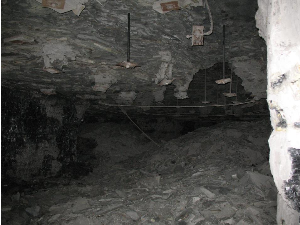
Figure 22: Progressive spalling between roof bolts in a moisture-sensitive roof shale.
