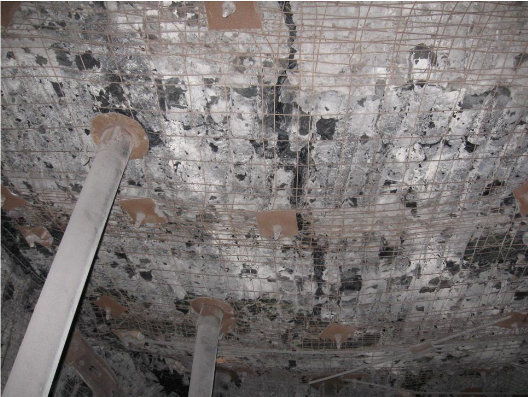
Figure 40: Tension crack in the entry center.
