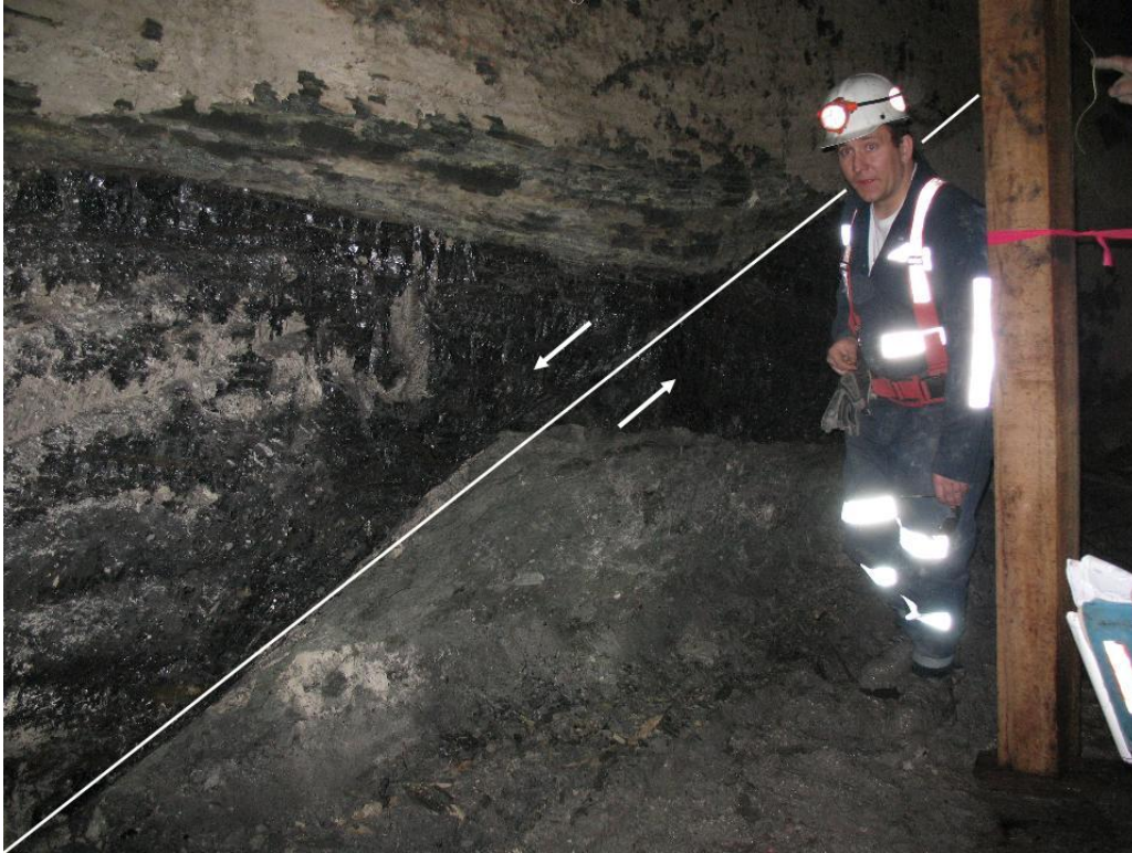
Figure 9: Normal fault causes roof damage in an Indiana coal mine.
