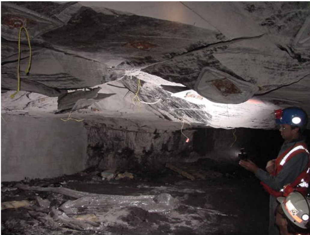
Figure 10: Slickensided failure planes cause hazardous roof conditions.
