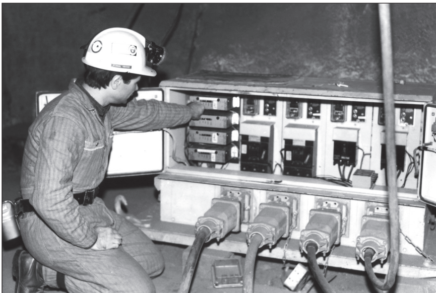
Figure 6. Sensitive AC GFR's installed in Safety Research Coal Mine
