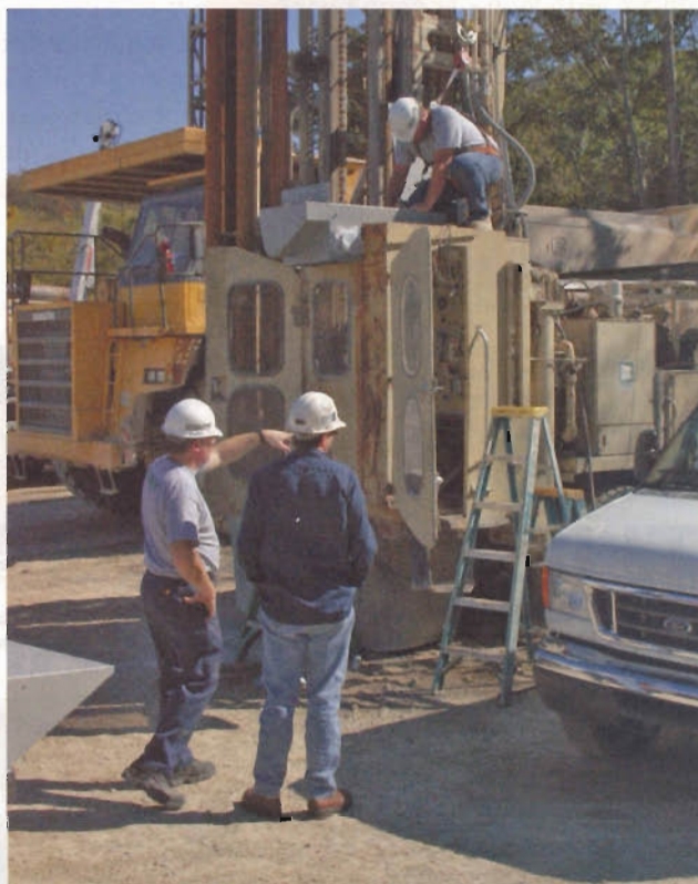
These drill operators are busy installing a new unidirectional filtration and pressurization system.
