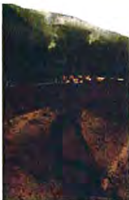
Crater and damaged roadway
