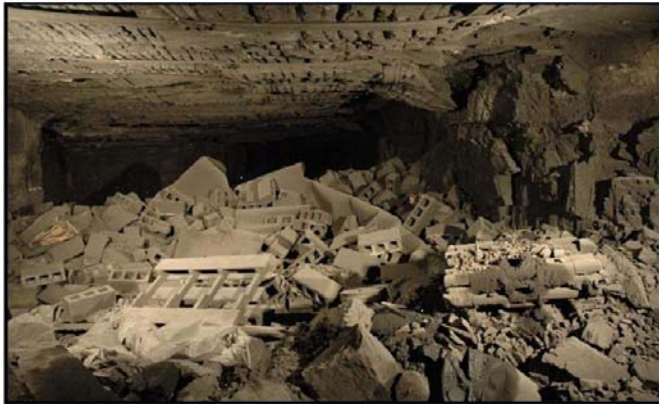
Figure 2. Debris from stopping near explosion (MSHA 2006).
