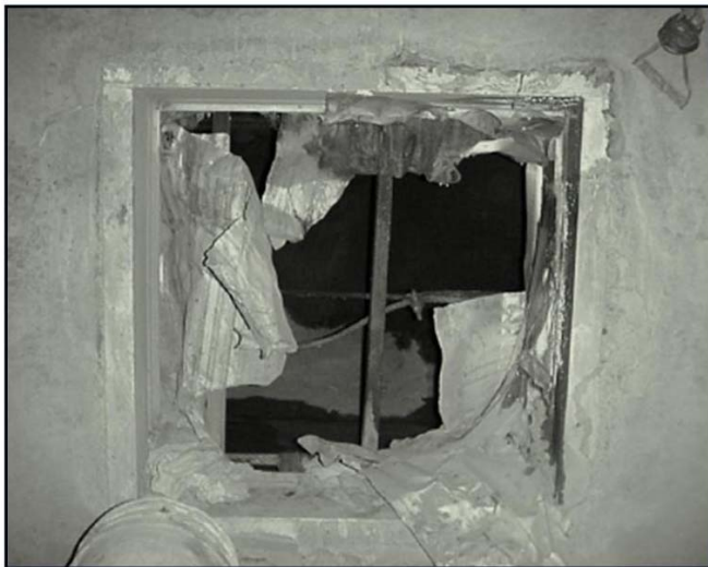
Figure 3. Corrugated, galvanized steel sheeting after explosion (MSHA 2003).
