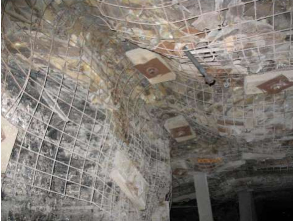
Figure 18: Full screening down the rib protects exposed corners and prevents rock falls.
