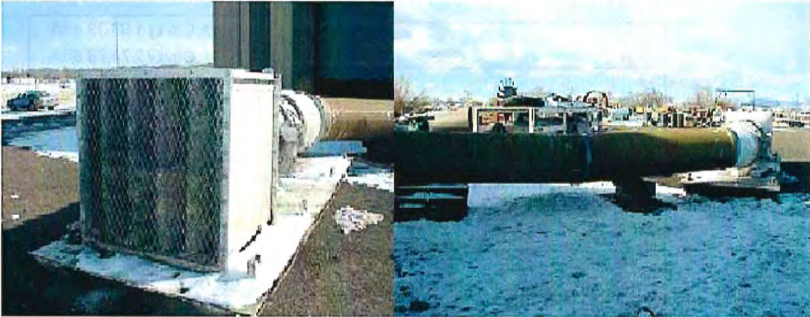
Figures 9 and 10 - Fan and Ductwork from March 2002 Experiment
