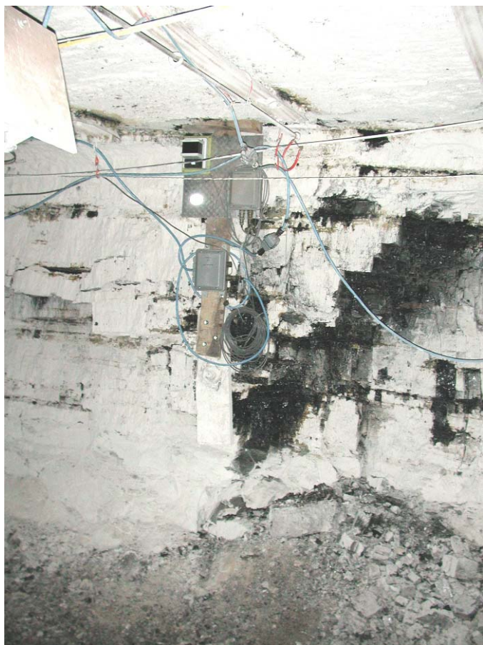
Figure 8. The Beam transmitter mounted on the rib in the haulage way.
