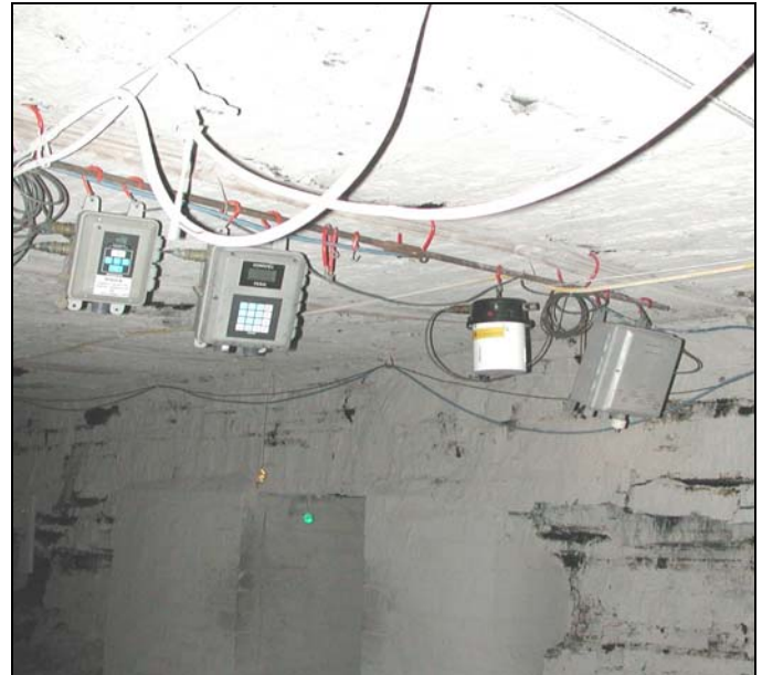
Figure 1. The smart mine fire sensors in the main haulage way, from left to right: Conspec CO Monitor, Conspec Diesel Discriminator, Becon Smoke Detector, and NIOSH MOS unit.
