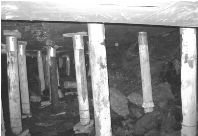
Figure 3. Engineered yieldable timber props equipped with active prestressing mechanical devices used as breaker line supports.
