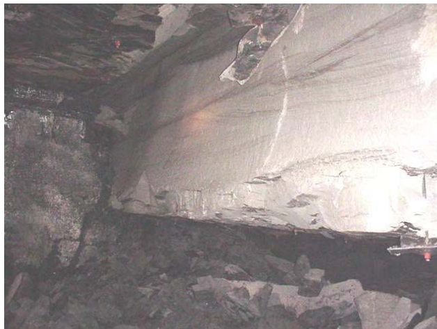
Figure 8.—Damage caused when open entries were subsided.
