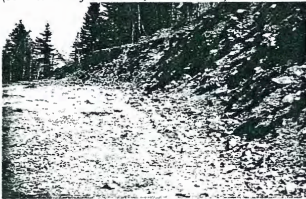
Figure 3. Minor raveling along a bench face
