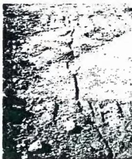
Figure 6. Example of tension cracks.
