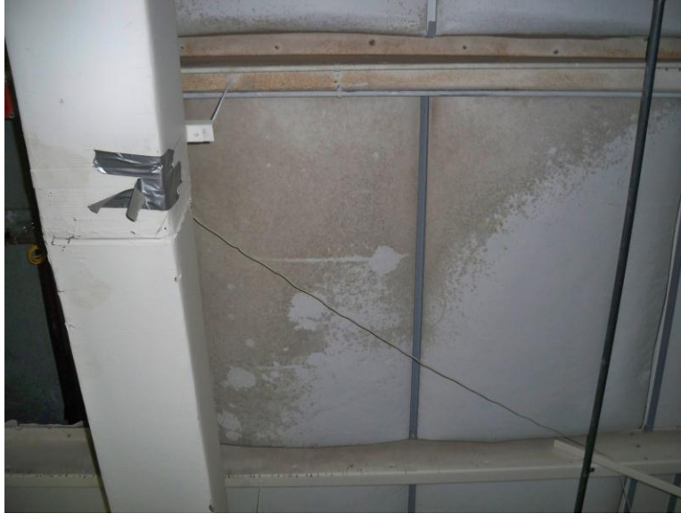
Figure 2: pPVC material affected by fungal growth
