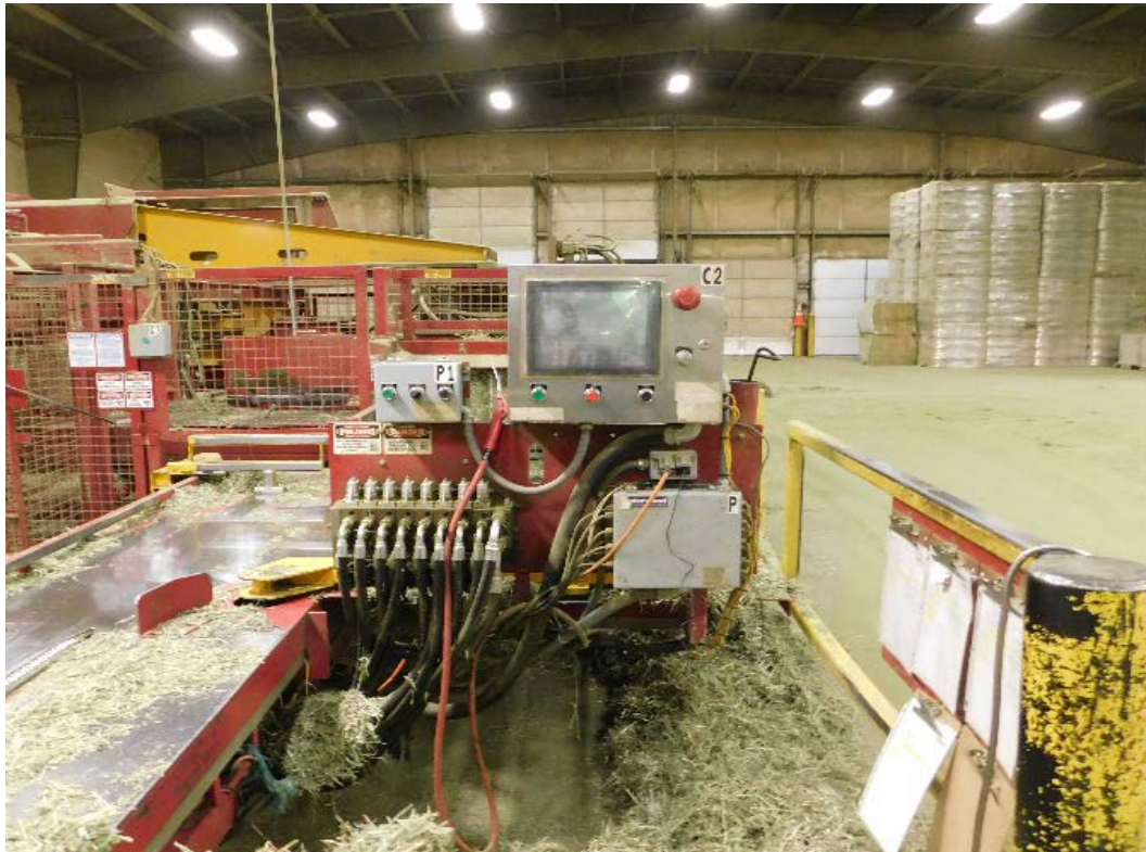
Photo 6: Operator's station with touchscreen interface panel.
