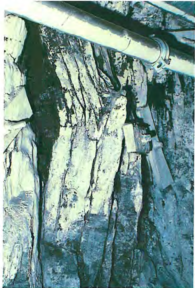
Figure 2. Photograph illustrating rib failure by buckling.
