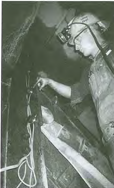
Figure 6. Load-cell washers installed on one side of control gate support bolts.
