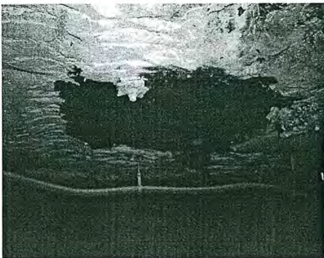
Figure 2. Skin failure in supported roof.
