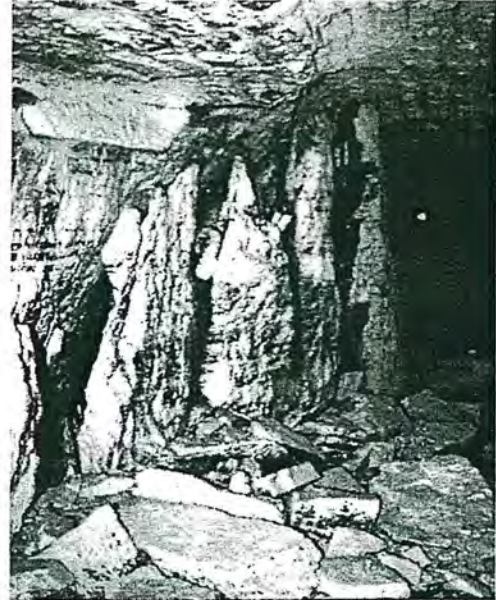
Figure 3. Skin failure of unsupported rib.
