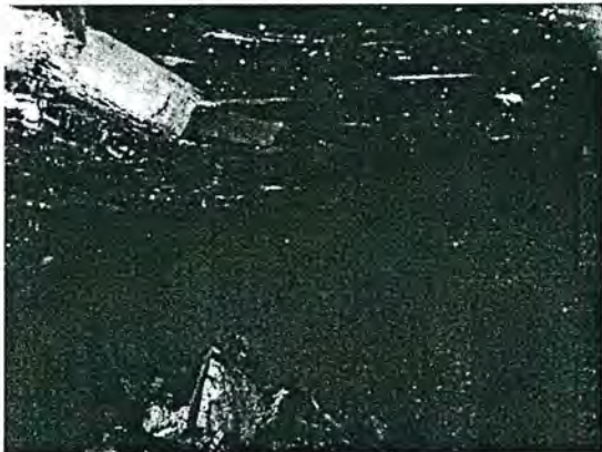
Figure 1. Skin failure of unsupported roof.
