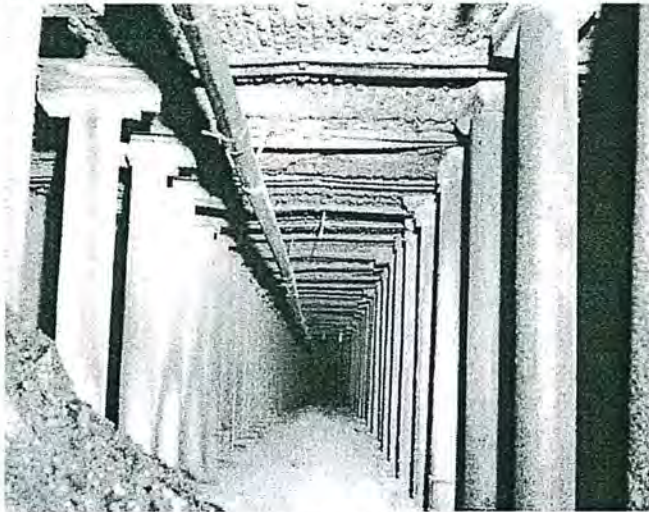
Figure 12a. Outby area supported by Propsetter support.
