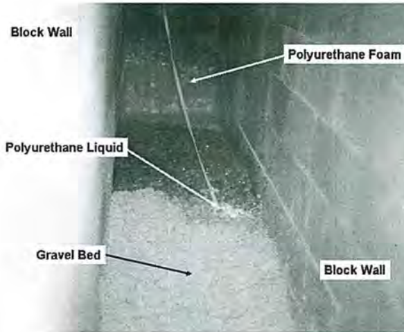
Figure 10.: Photo of inner core of Mine Seal No.2 during addition of polyurethane resin.
