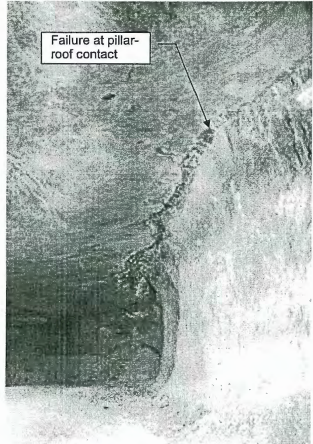
Figure 1. Photograph showing failure at pillar-roof contact after loose rock has been removed and roof has been re-supported.
