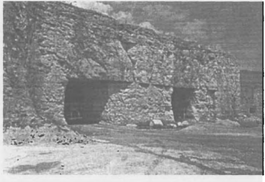
A smooth roof line produced by a persistent bedding-plane lamination within the limestone roof beam.
