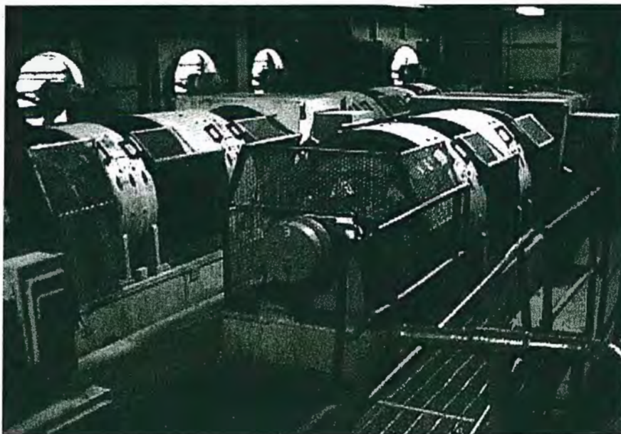
Example of a M/G set in back of dragline house.
