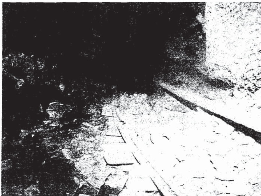
Figure 8 Burst Damage in Lateral, Lucky Friday Mine.
