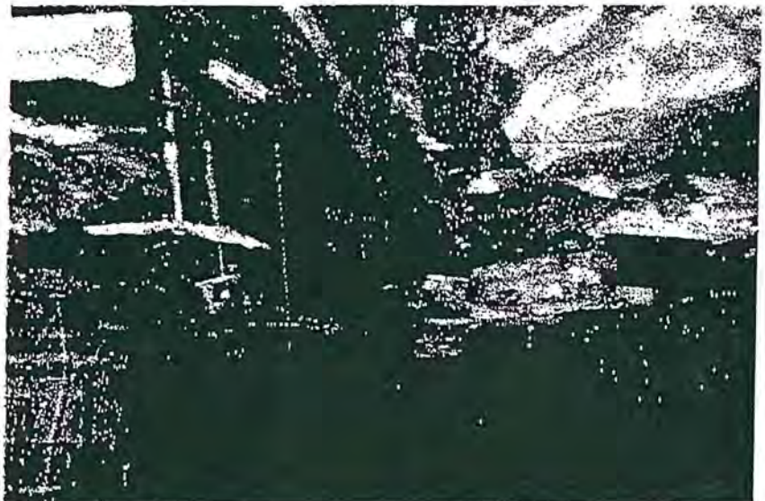
Roof failed due to break up of roof strata along randomly oriented slickensides.
