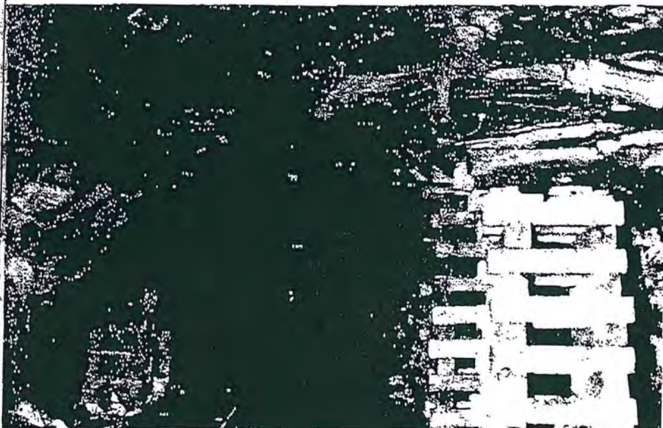
A highly laminated roof rock weathers around the bolt's bearing plates.
