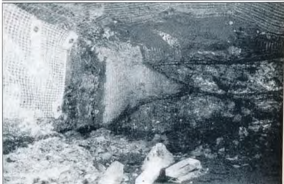
Fig. 8. Typical thrust fault found in No. 3 main development entry.
