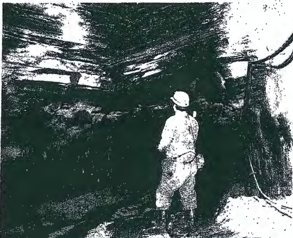
Researchers now believe that cutter roof formations, such as the one shown above, are the result of horizontal stress.
