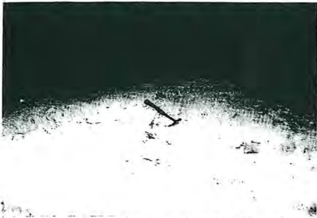
Figure 12. Floor heave experienced in E15 panel.
