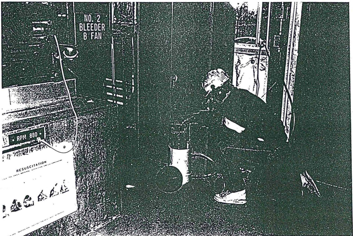
Figure 4B.-Photo of copper tubing from bleeder fan housing connected to AGS system in equipment room.
