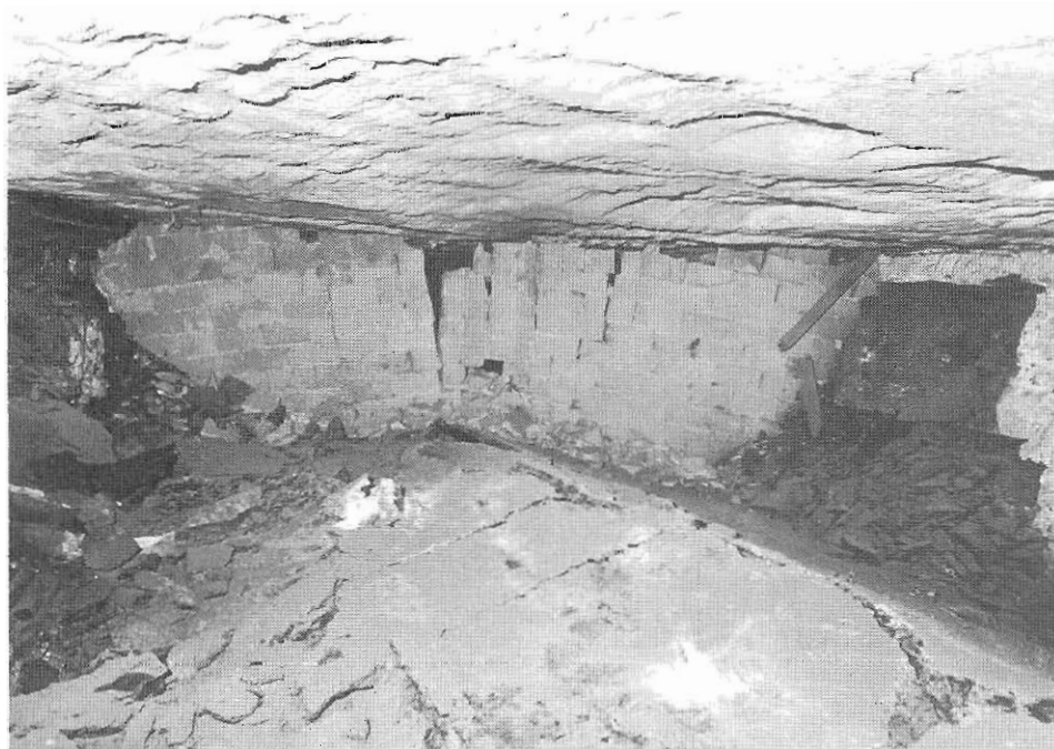
Fig. 2 — Stopping destroyed by floor heave, Blue Creek No. 5 Mine
