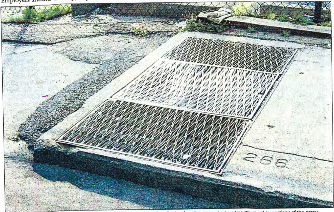
Know the intended load capacities for grates and have registered professional engineers conduct routine structural inspections of the grates.
