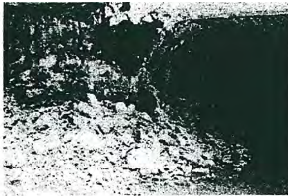
Figure 6-12 Rib's sloughing at 2200 ft deep
