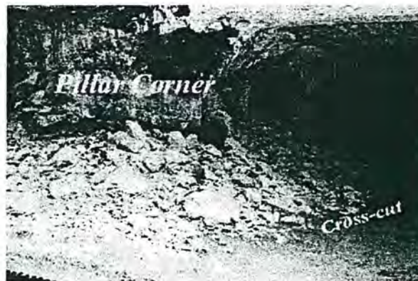
Figure 5-4 A photo for a failed pillar corner
