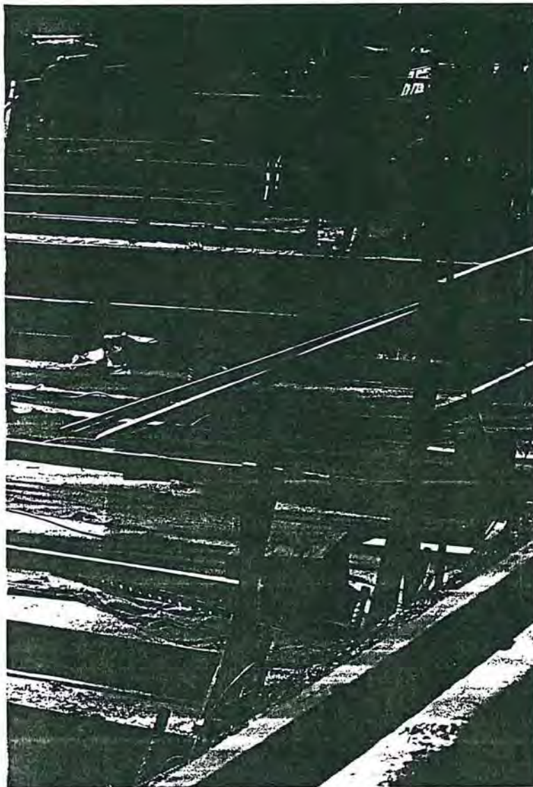
16: Below: Ironworker platform with "SAVE" painted on it and stored near Ironworkers' trailer; rope handle broken
